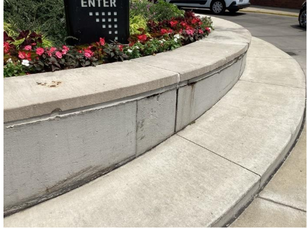
Planter wall cracks
