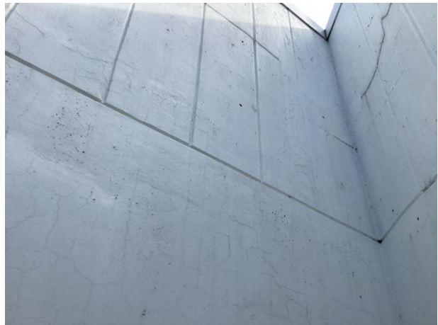
Cracks at penthouse structure
