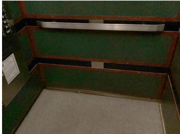
Elevator cab finishes for passenger elevator
