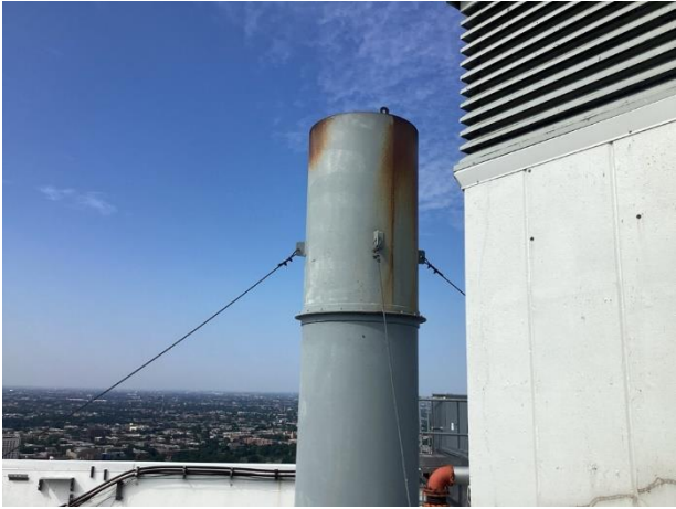
Boiler stack rust
