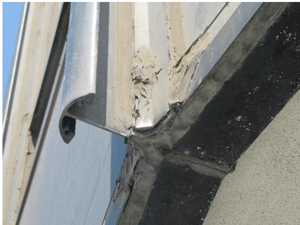
Sealant cracks at vertical mullion base
