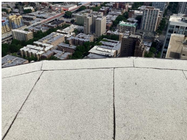
Perimeter sealant deterioration at tower roof
