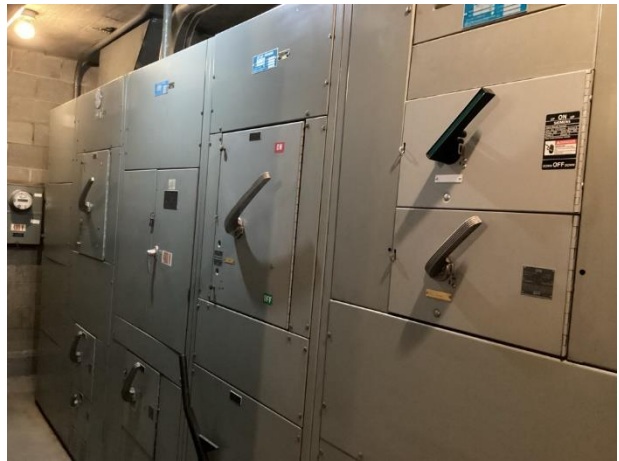
Electrical system main panels
