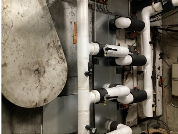
Air handling unit serving hallways (S2)
