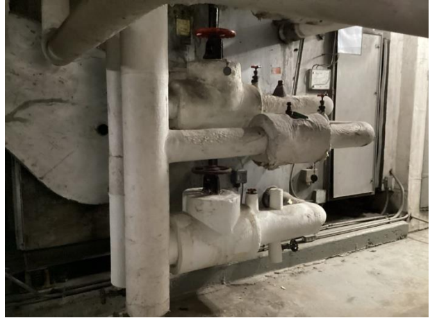
Lobby air handling unit
