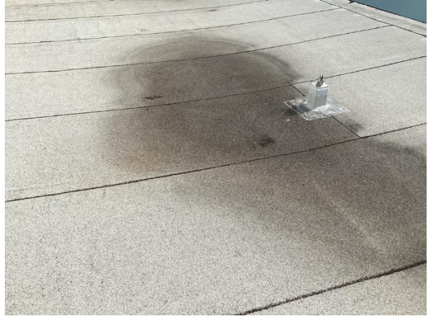
Depression at tower roof
