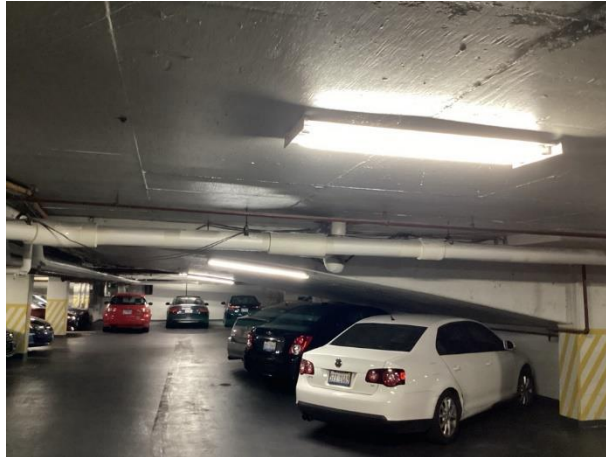
Garage light fixtures
