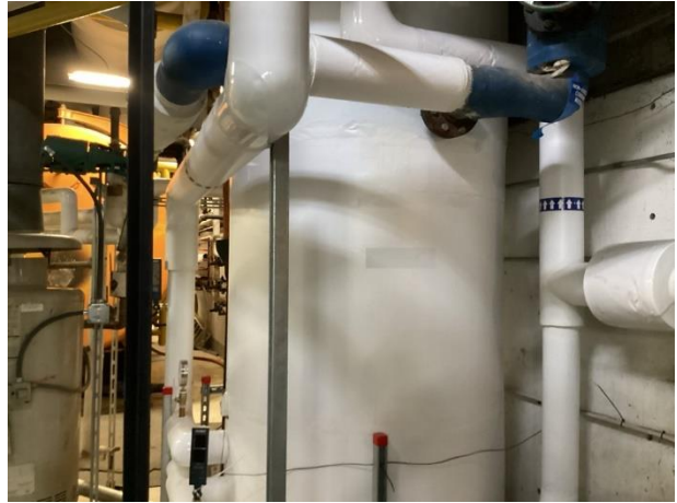
Low rise residential domestic water storage tank
