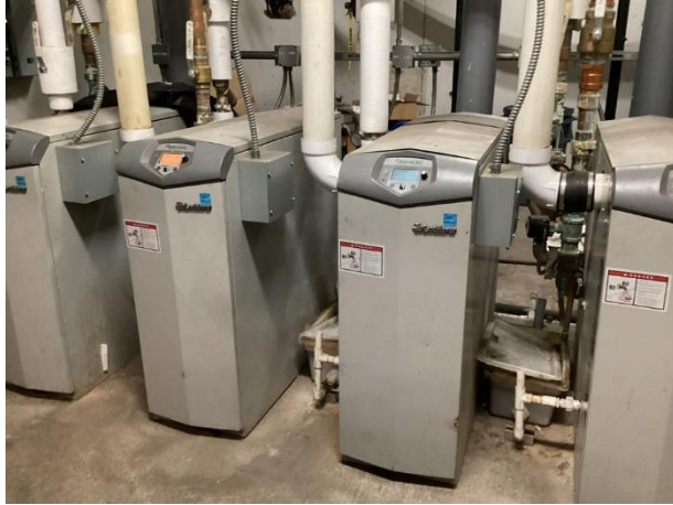
High zone domestic water boilers
