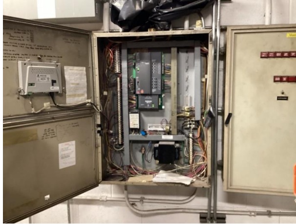
Main panel for heating system
