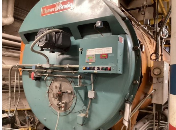
Building heat boiler
