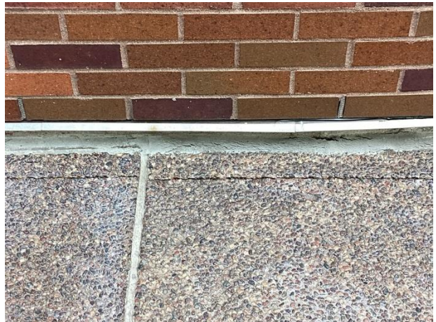
Joint deterioration at plaza
