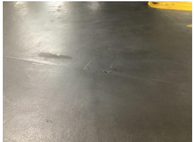
Traffic coating damage
