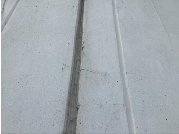
Crack at joint at penthouse structure
