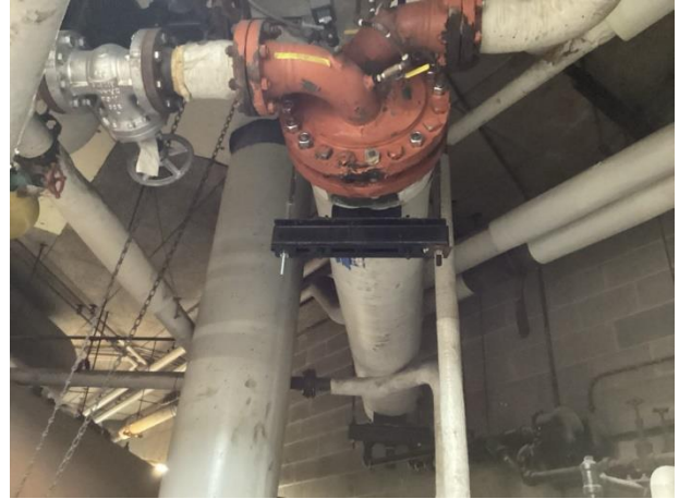
Perimeter heat exchanger
