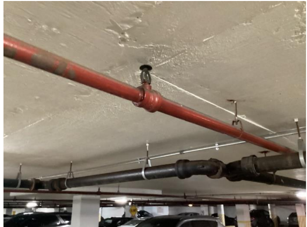
Fire suppression system at head
