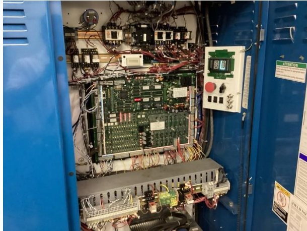
Low rise elevator controls
