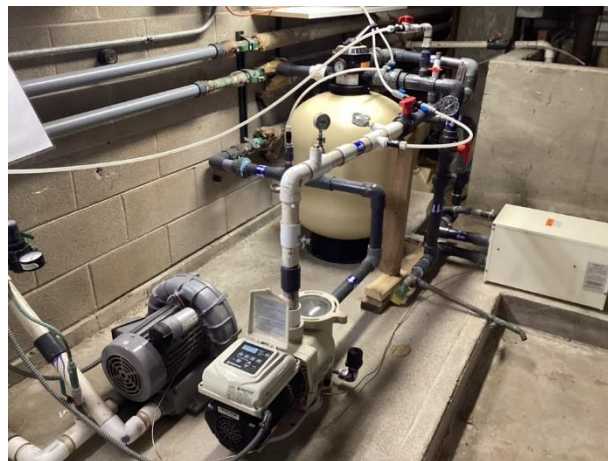
Spa mechanical equipment
