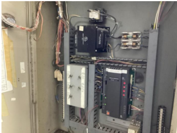
Building automation system panel
