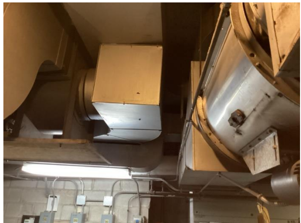
Basement air handling system fans
