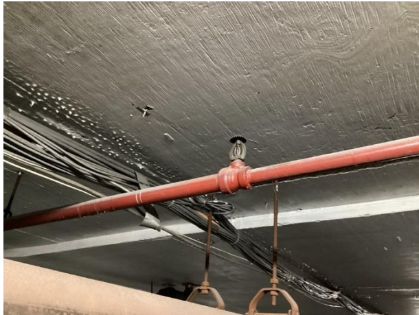
Fire suppression system at head
