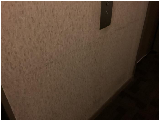
Dated wall covering
