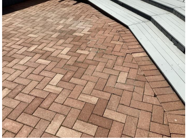
Paver settlement and cracks at 2nd floor roof
