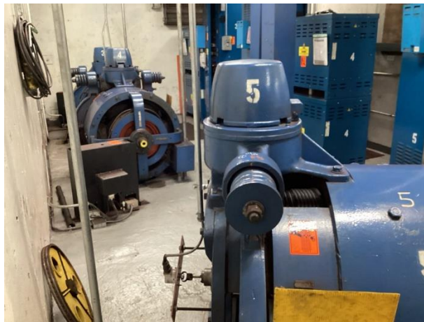
Traction elevator hoists and motors
