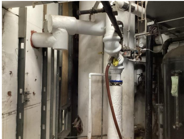
Penthouse domestic water storage tank
