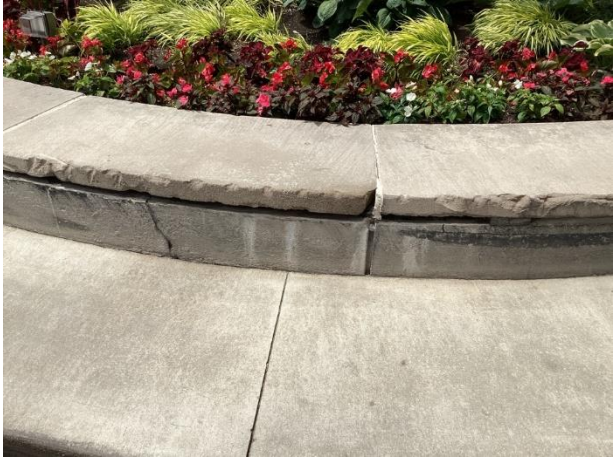
Planter joint deterioration
