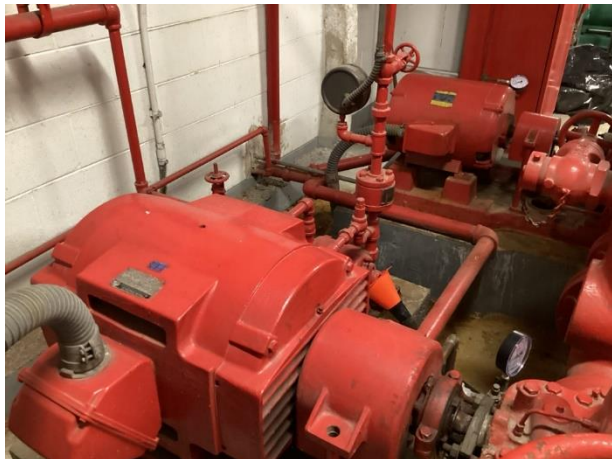
Fire suppression pumps
