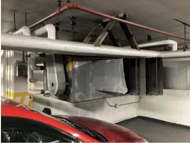
Garage air handling unit
