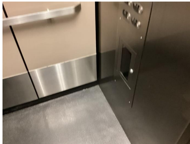
Hydraulic elevator cab finishes
