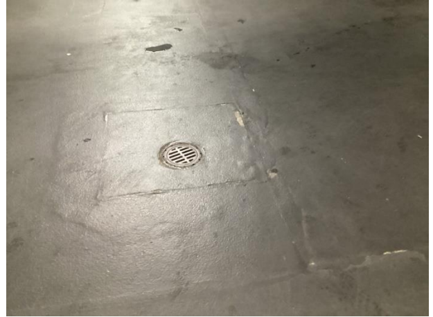
Traffic coating damage
