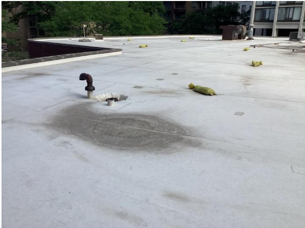
Northwest 2nd floor roof at depression
