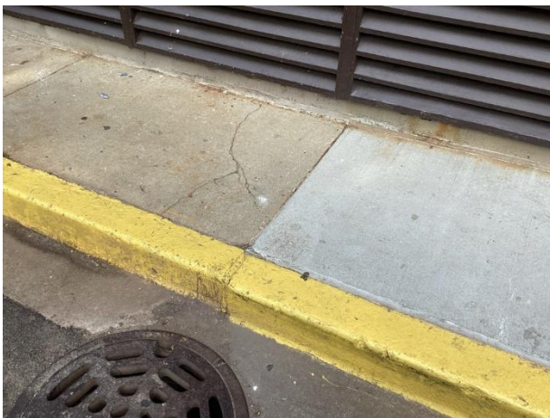
Crack at sidewalk
