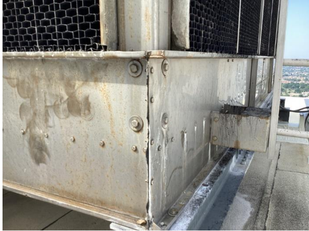
Cooling tower at previous seepage
