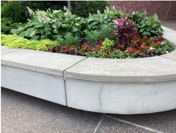
Crack at planter wall
