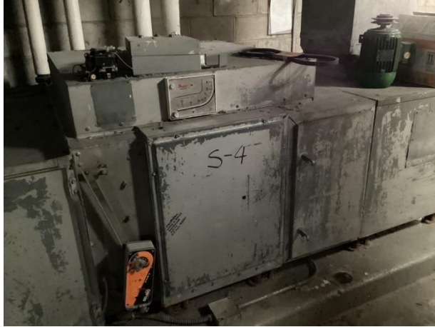
Laundry room air handling unit
