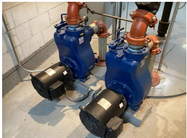
Sewage ejector pumps
