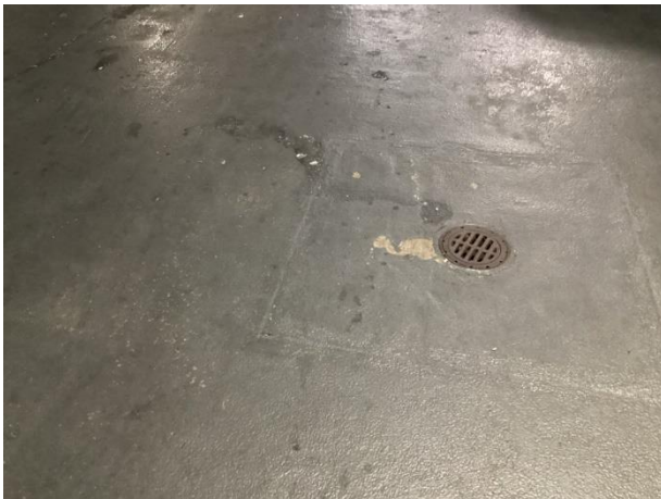
Traffic coating damage
