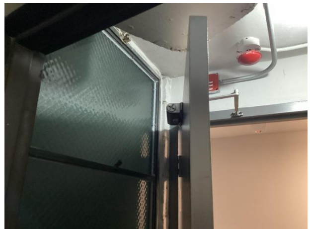
Smoke damper system
