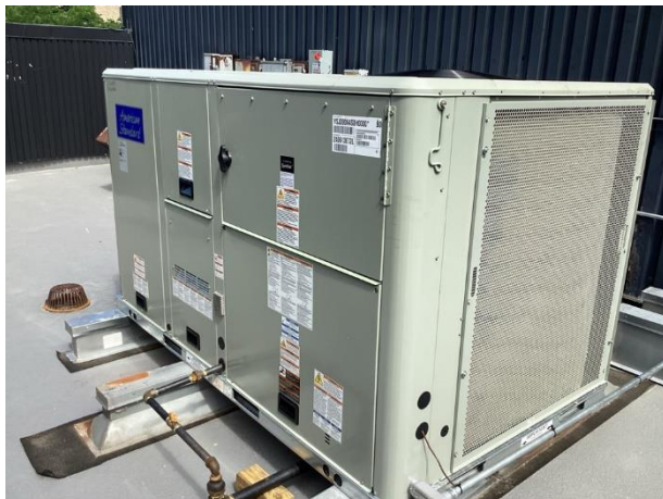
Racquetball court air handling unit
