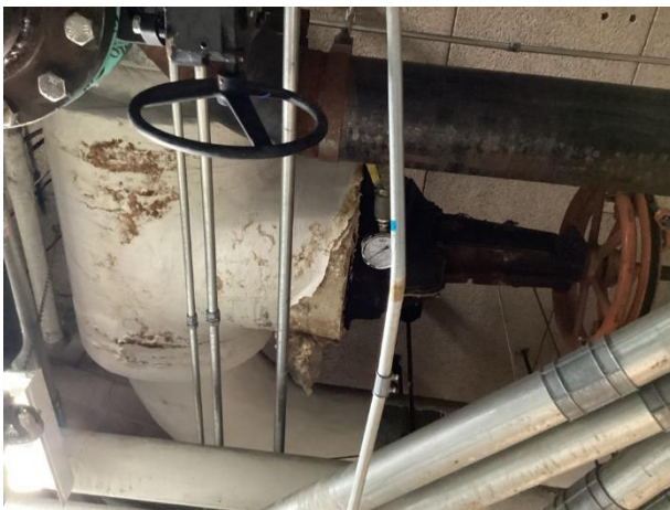
Chiller room large diameter valves
