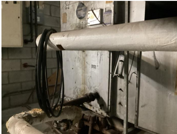
Mall air handling unit
