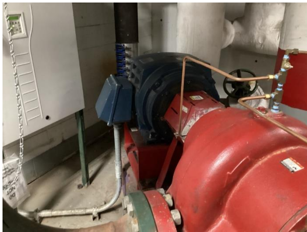
Cooling tower pump
