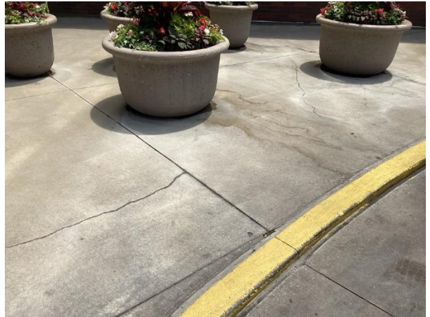
Cracks at concrete
