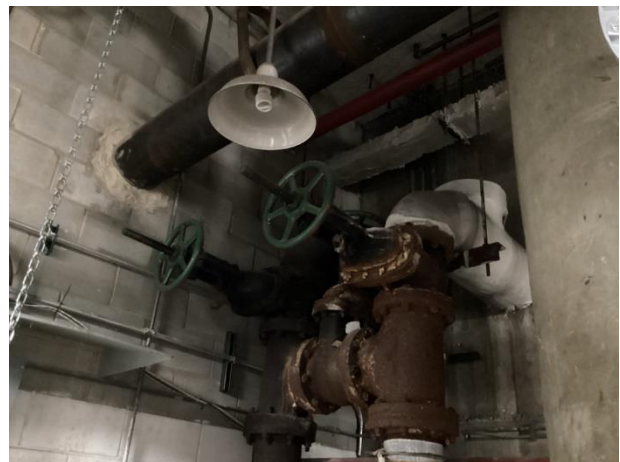
Main water connection large diameter valves
