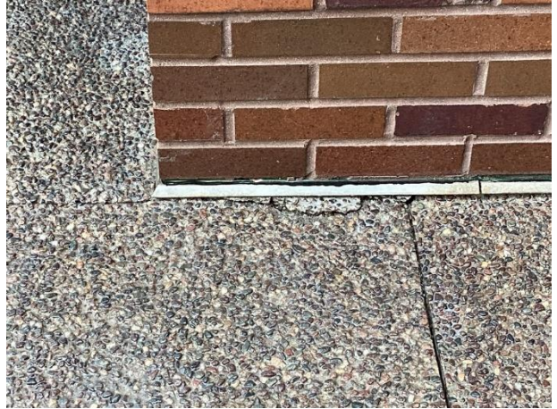
Crack at perimeter at plaza
