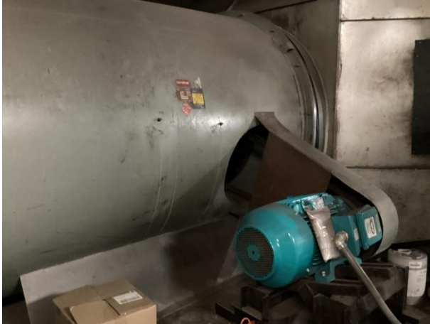
Recently replaced motor at exhaust fan
