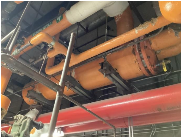
Pool heat exchanger
