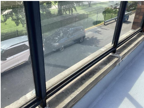
Glass damage at steel corrosion at 2nd floor east railing
