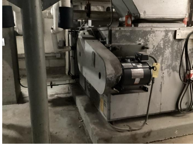
Party room air handling unit
