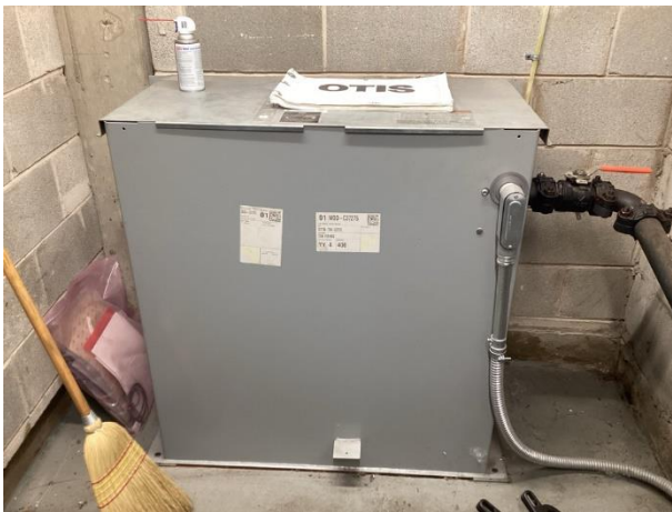
Refuse elevator power unit casing
