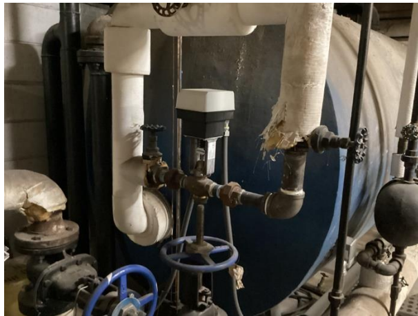
Feed water system
