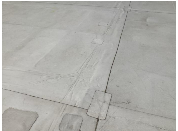
Patches at northwest 2nd floor roof
