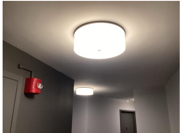
Recently replaced light fixtures
