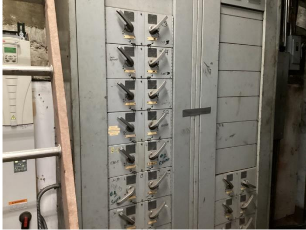
Motor control center
