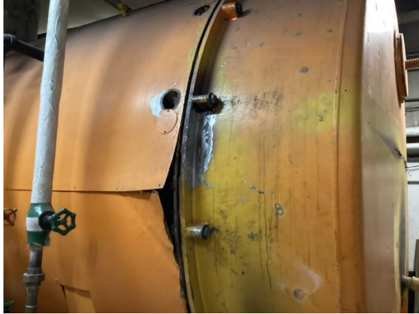
Building heat boiler at shell
