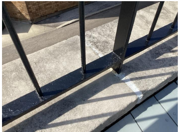
Rust at inset post at 2nd floor railing
