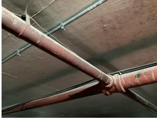
Fire suppression system at main and branch pipes
