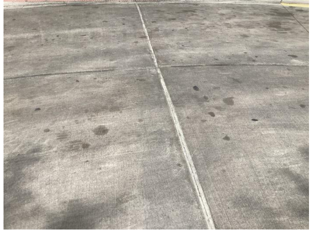
Joint deterioration at driveway
