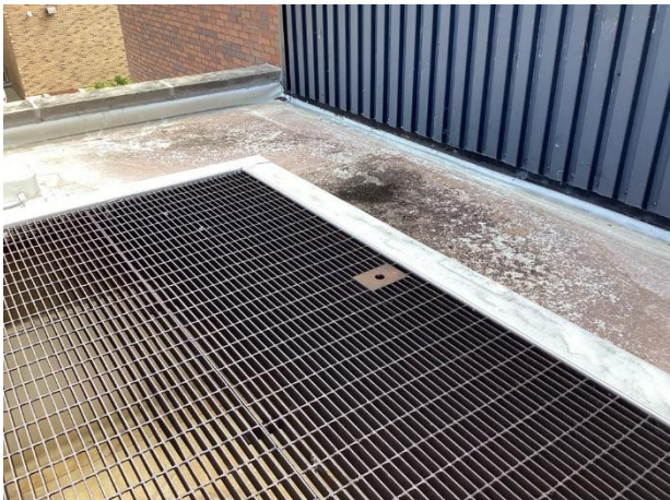
Northwest 2nd floor roof at lack of drainage
