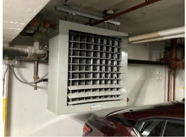
Garage unit heater
