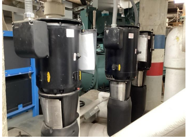
Domestic cold water pumps
