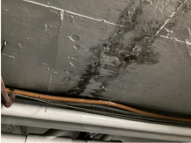
Evidence of past water infiltration beneath the plaza
