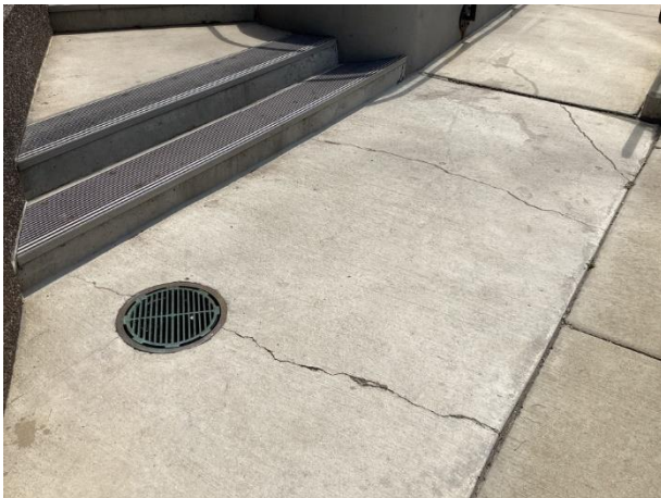
Cracks at concrete
