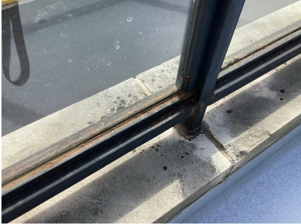
Steel corrosion and inset post at 2nd floor east perimeter
