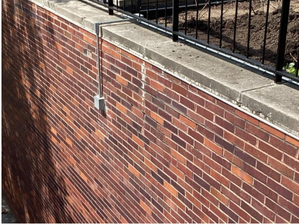
Masonry crack and spall
