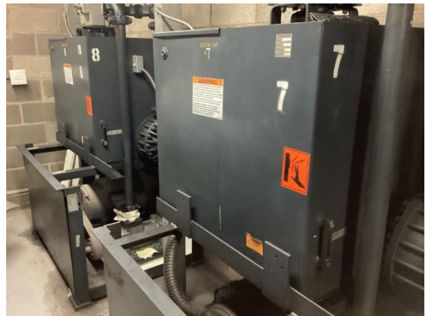
Hydraulic elevator equipment for mall and garage
