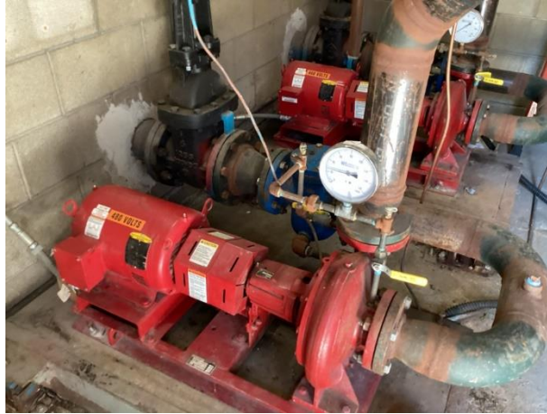
Cooling pumps for commercial
