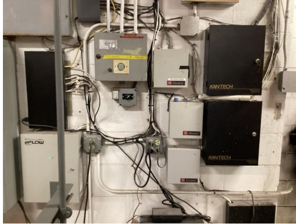
Fob system control panels
