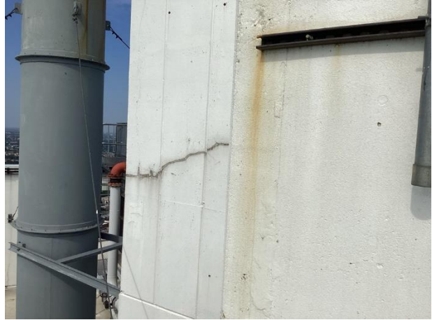
Cracks at penthouse structure
