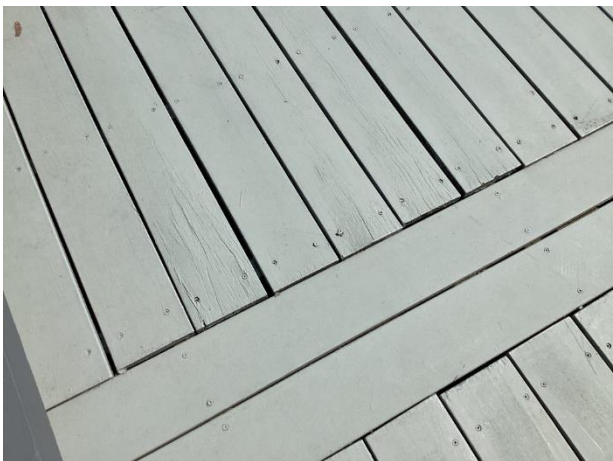
Weathered wood decking at 2nd floor roof
