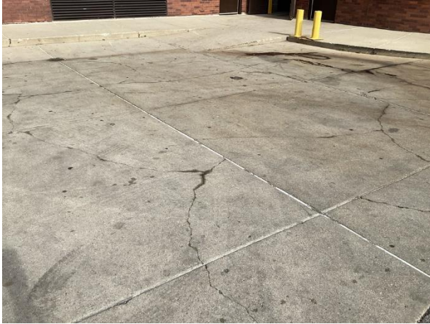
Service dock pavement cracks
