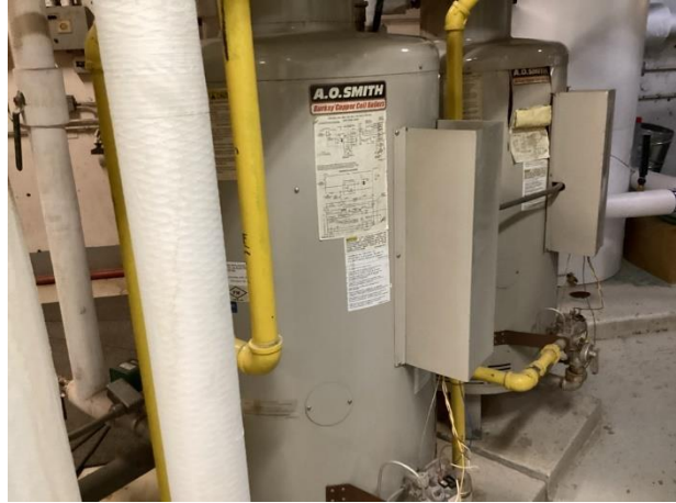
Commercial domestic water boilers
