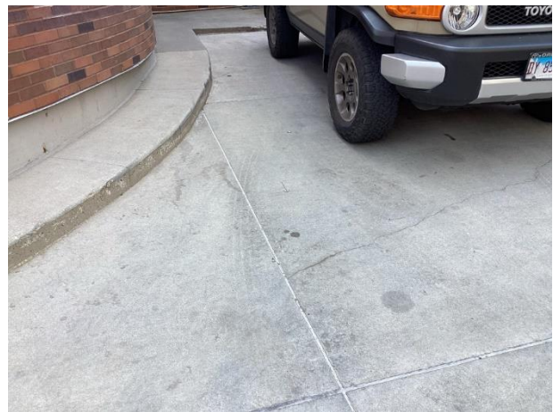
Service area pavement cracks
