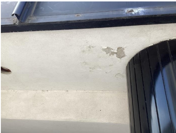
Soffit finish damage
