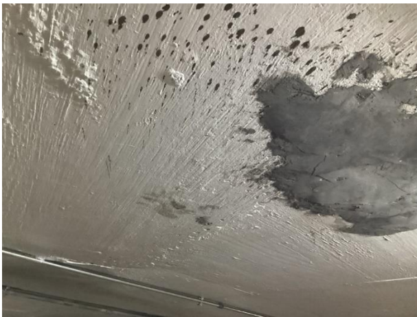
Crack at repair beneath elevated floor
