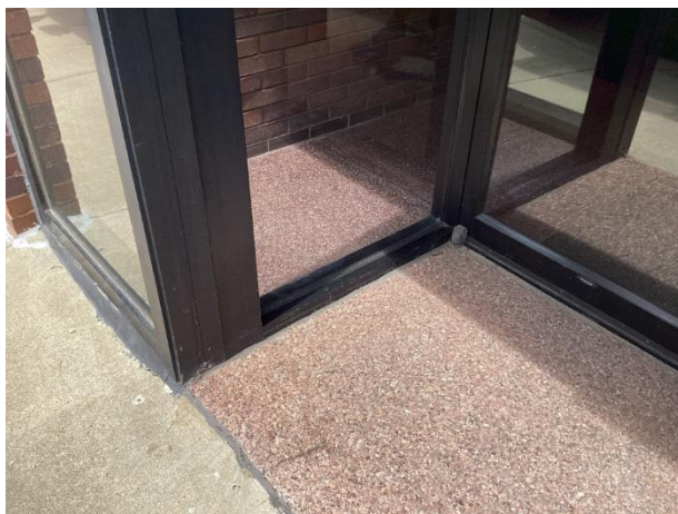
Window and door system at entrance at mall
