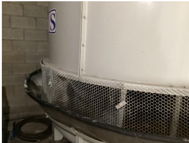
Commercial cooling tower
