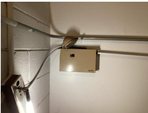
Emergency battery pack fixture
