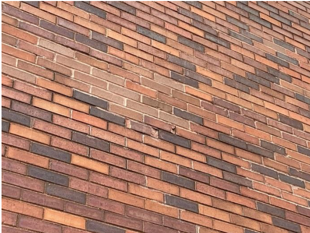
Masonry spall and joint deterioration
