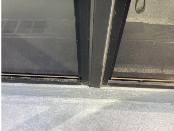
Walkway window system at joint sealant deterioration
