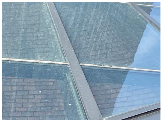
Skylight at joint sealant deterioration
