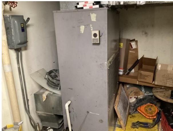
Air handling unit for low rise passenger elevator room
