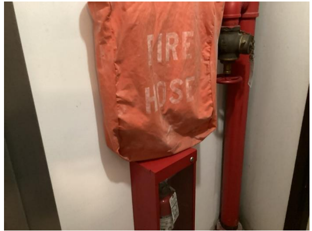
Fire hose and extinguisher
