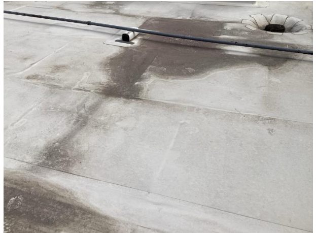
Northwest 2nd floor roof at depressions
