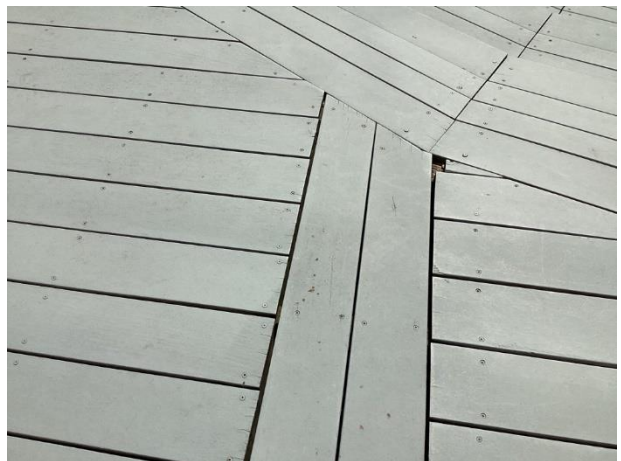
Weathered wood decking at 2nd floor roof
