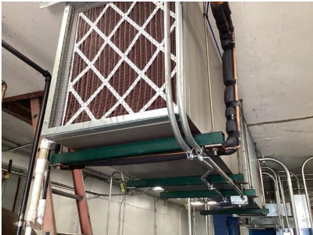
High rise elevator room air handling unit
