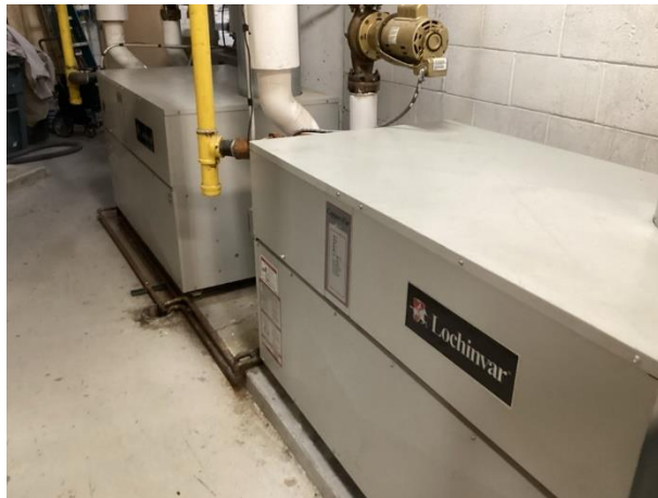
Low zone domestic water boilers
