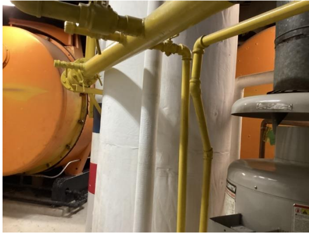
Commercial domestic water storage tank
