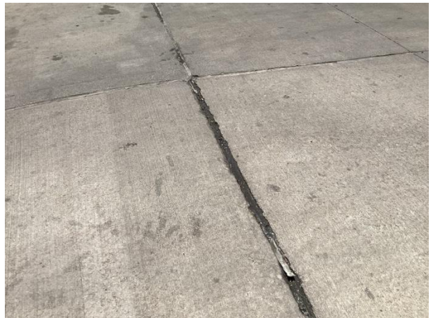
Driveway joint deterioration
