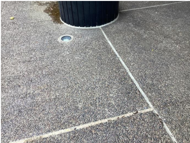
Joint deterioration at plaza
