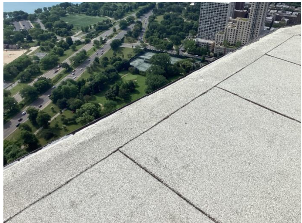
Perimeter sealant deterioration at tower roof
