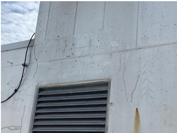
Cracks at penthouse structure
