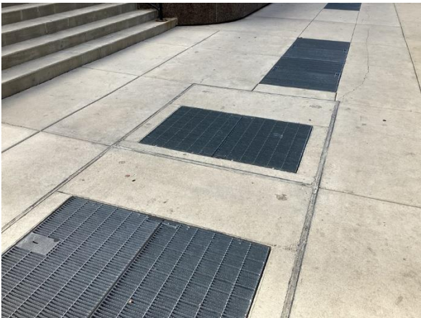
Electrical utility vault at west perimeter
