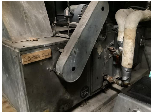
Pool air handling unit
